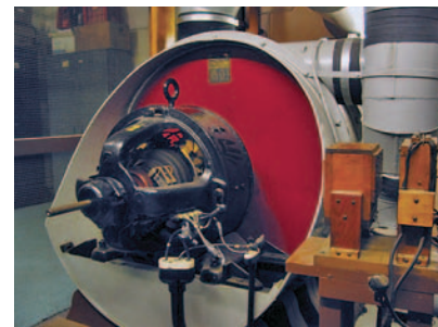
One of the blowers at Woolsey Hall
