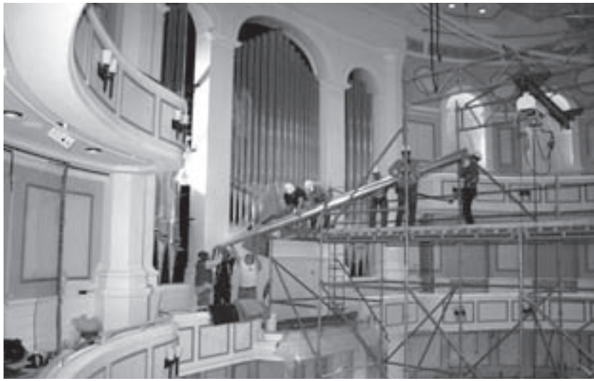
Goulding & Wood façade, Palladium Concert Hall, Carmel, Indiana
