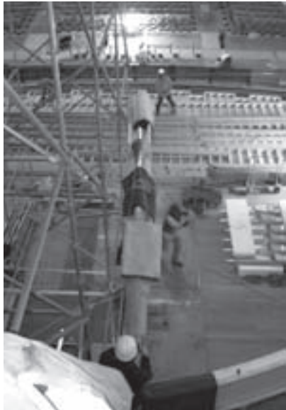
Goulding & Wood façade, Palladium Concert Hall, Carmel, Indiana
