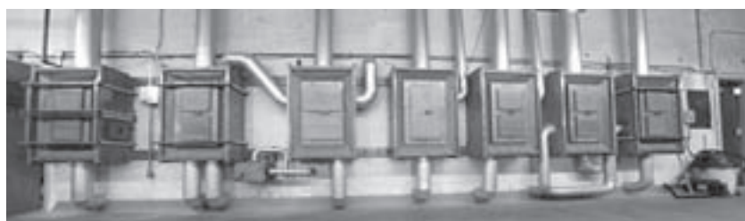
The array of reservoirs for the right stage chamber on the Midmer-Losh organ
