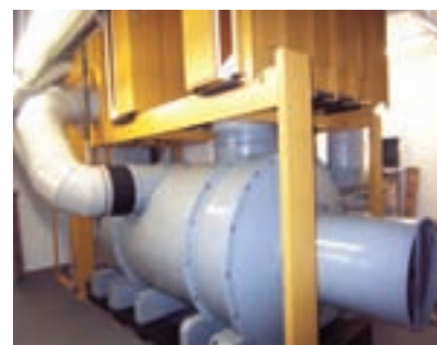
The reconditioned, 30-horsepower, triple-outlet Spencer blower
