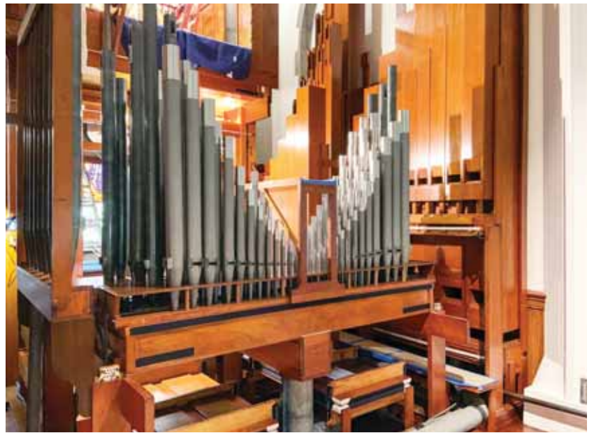
Great main pitman chest during installation
