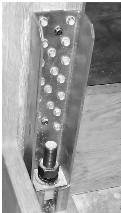
Anti-seismic anchors: twelve steel anchors are bolted through the concrete floor with 7/8" threaded rods (photo credit: Noack Organ Co.)
