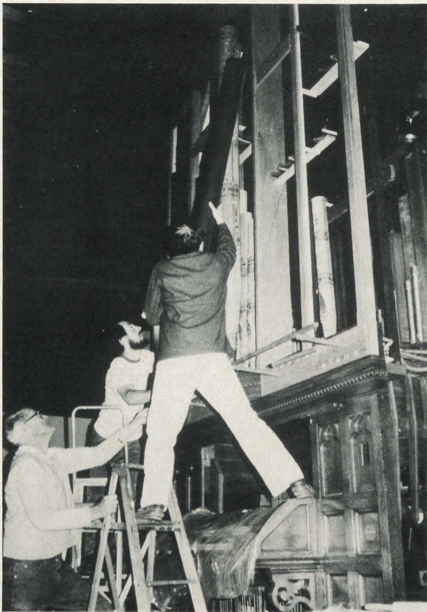
Left to right: Messrs Wulbrandt, McNeil and Fruhauf install the façade pipes.
