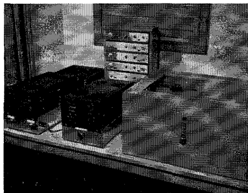
THE EQUIPMENT ROOM. Shown here are the control circuits and the memory mechanism. The power amplifiers are located below.
