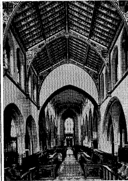
The ceiling over the choir, recently decorated, shows up vividly in the view below.
