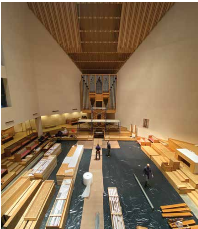
Pipework packing by the Organ Clearing House, with fine silt visible on floor beyond edges of plastic covering (photo credit: Jared R. Stahler)
