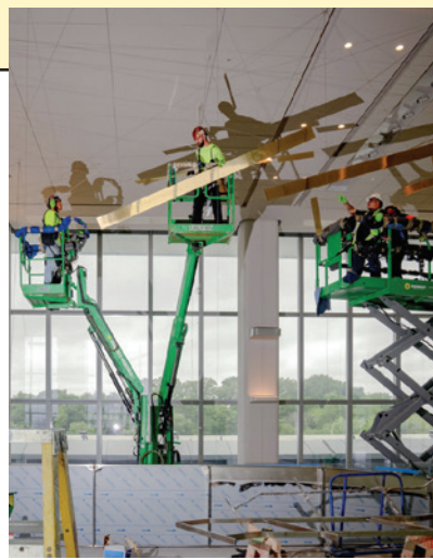
Orpheus and Apollo during its installation in LaGuardia Airport. The crew had to reassemble 188 metal bars, suspended at precise angles midair, from 444 wires attached to the ceiling. (photo credit: AMIR HAMJA/The New York Times/Redux)
