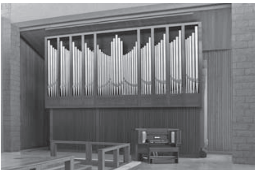
Day 8: The installation of the organ is complete and ready for tonal finishing.
