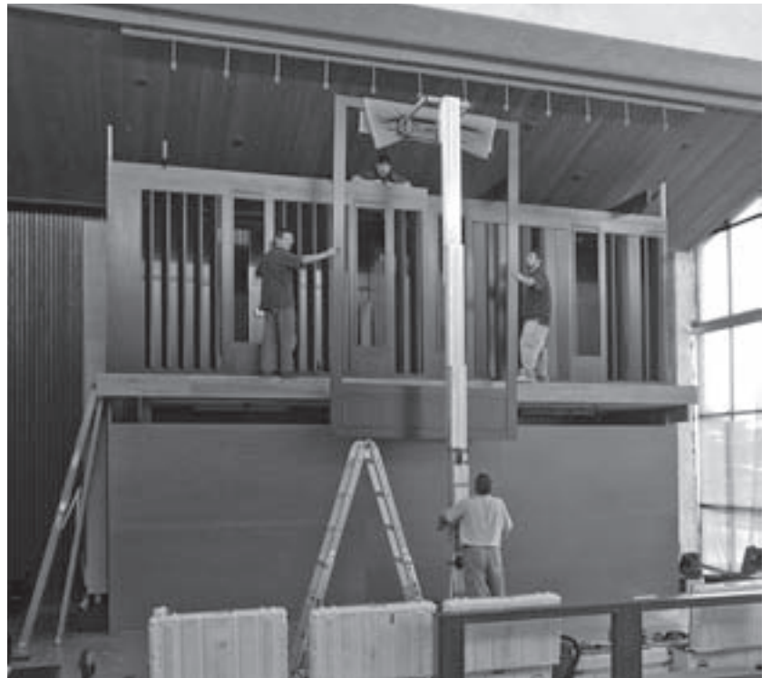
Day 4: With the winding components and blower all in place, the upper casework is hoisted into position.
