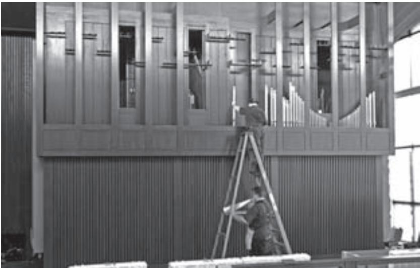
Day 6: After the initial testing of the winding and wiring systems, the pipes are installed. The two ranks visible here are part of the Open Diapason and Harmonic Flute.
