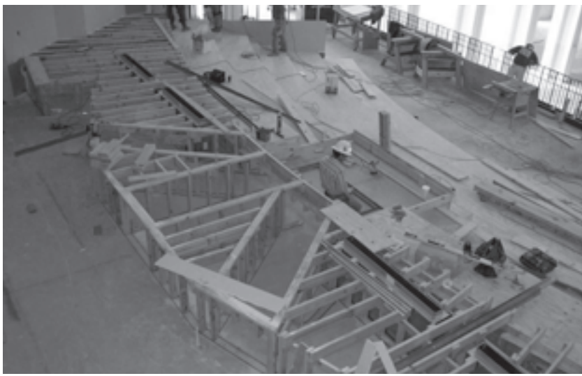
Construction of choir risers with channels for the tracker actions (photo by Martin Ott)
