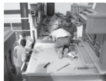
Installation of steel beams to support new Rückpositiv (photo credit: Ron Turner)
