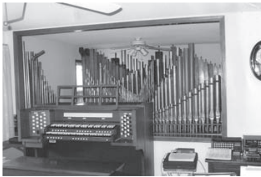
A very tight installation in a 10' x 12' bedroom with opening into living room in DeKalb house
