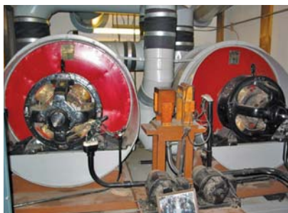
Woolsey Hall blowers
