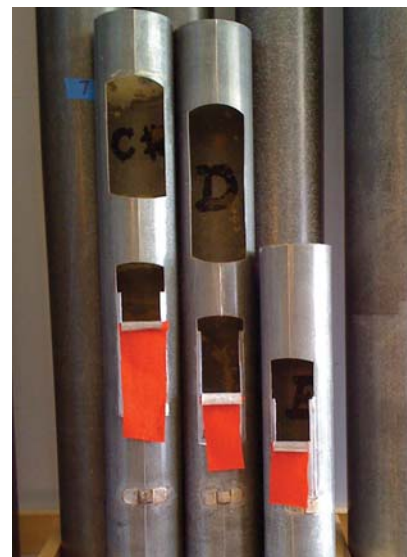
New spotted metal tuning inserts installed on stripped façade pipes prior to finishing
