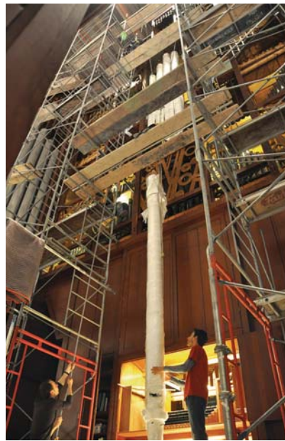
Installation of the five new façade pipes of the Montre 16 (photo credit: Robin Côté)
