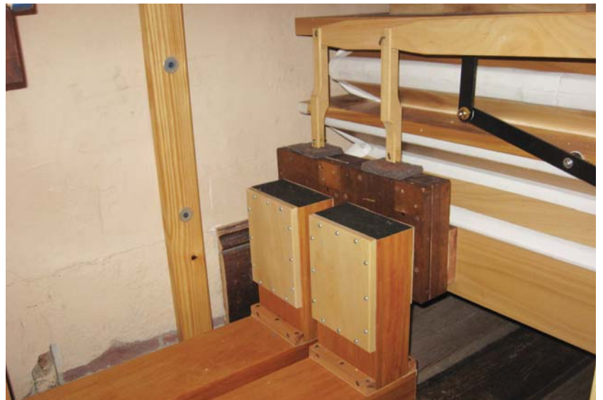
5. Ducts and vents (Photo credit: Nicholas Ringwald)
