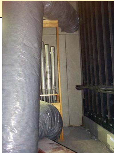
9. HVAC ducts routed through organ chamber, obstructing tone and preventing tuning or maintenance access
