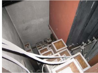
10. Building system cables routed through organ chamber, laying on pipes and preventing reliable tuning or access to organ parts
