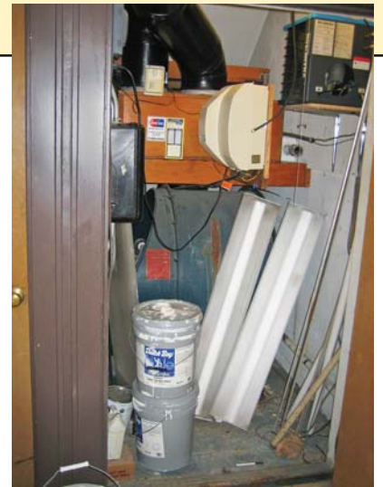
12. Blower room used as building storage space; conditions are dangerous, dirt laden, and organ air intake is obstructed.
