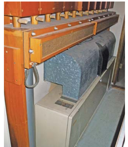
13. HVAC equipment within organ chamber generating excessive heat prevents tuning stability
