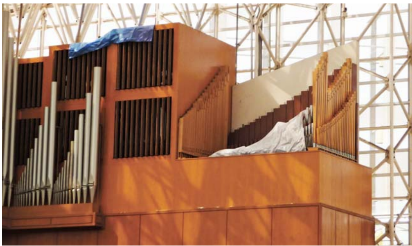
Gallery organ, prior to restoration. Several areas of the organ were temporarily protected to limit the damage from rainwater from leaks in the roof.
