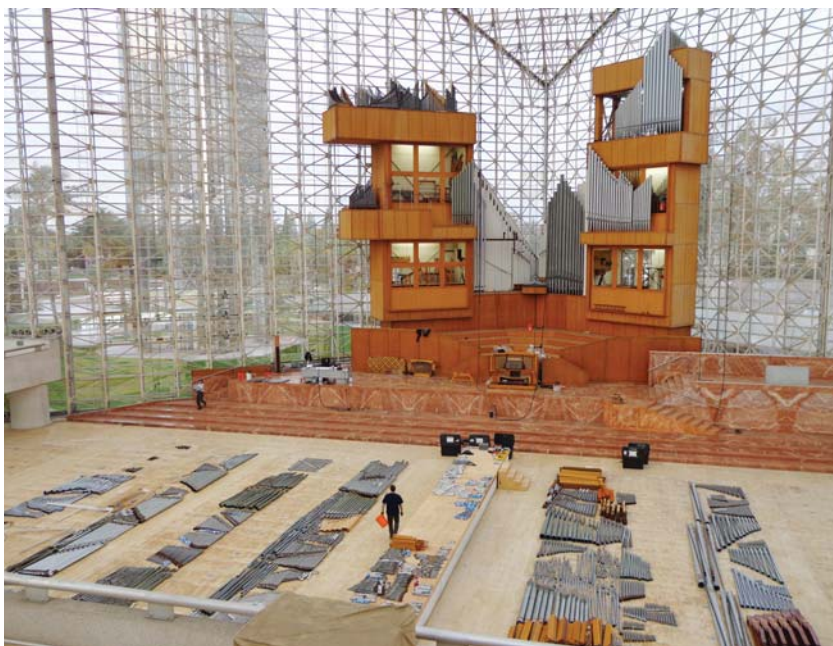
The organ's disassembly: all chairs have been removed from the cathedral floor and pipes are being carefully stored over the entire floor area, waiting to be packed.
