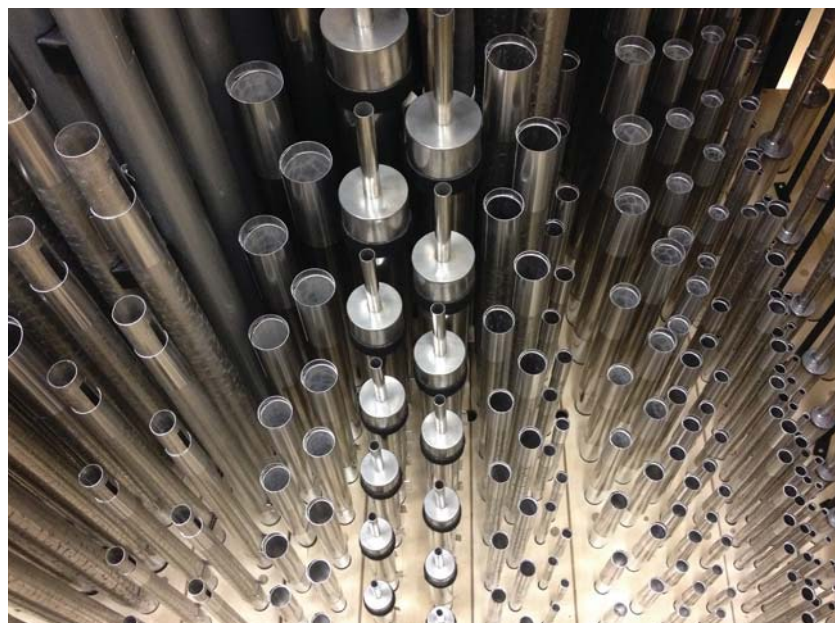
View of Great pipework
