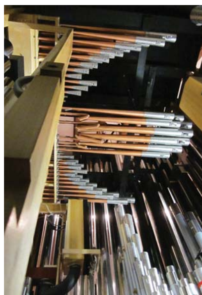
View of Pontifical Trumpet looking up from the Great/Pedal service ladder
