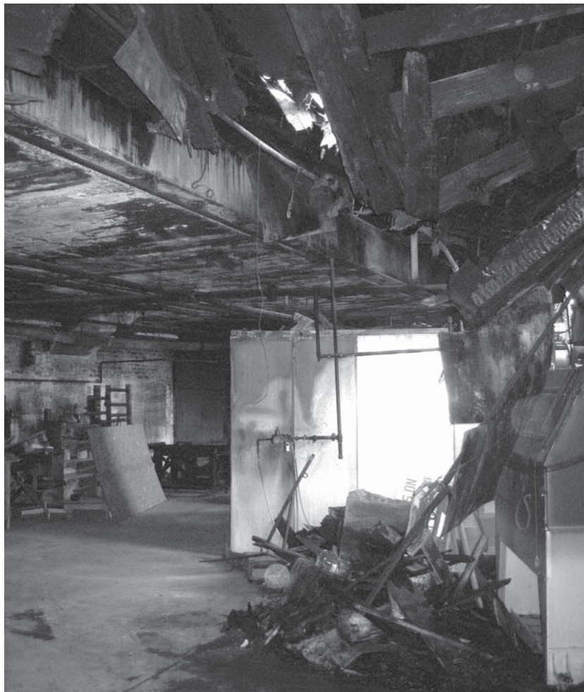
View from the loading dock area facing south toward the spray booth: in the center of the picture, the source of the January 2011 fire. Daylight at the top of the picture is from an open hole burned in the ceiling of the room.
