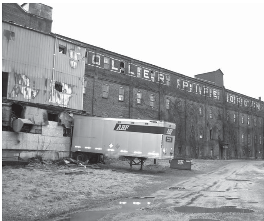
One of the ABF pup trailers is parked at the back loading dock, adjacent to the area of the January fire. Remnants of the spray booth exhaust fan hang out of the building. The back side of the original southwest building, dating from 1896, complete with Möller sign, clearly shows the extent of deterioration.
