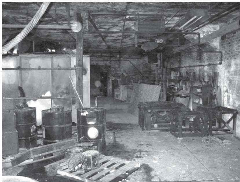
View of the burned area from the south, looking back toward the spray booth. Rick Morrison is taking notes and talking on the phone at the far end of the room.
