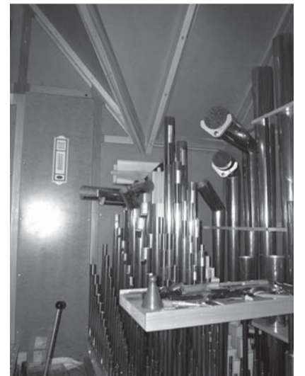
Hayes Barton organ Opus 39 showing complicated ceiling geometry
