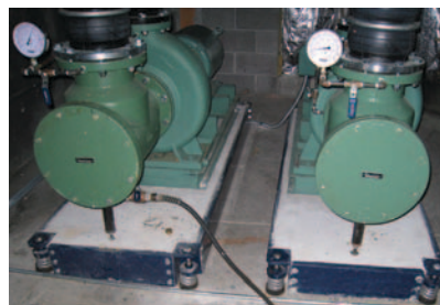
Unwanted noise and vibration can be controlled when equipment is resiliently mounted.
