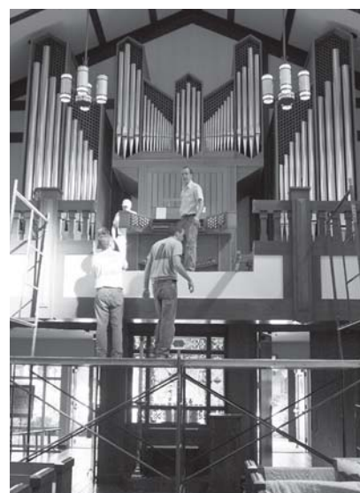
Installation of steel beams to support new Rückpositiv (photo credit: Ron Turner)
