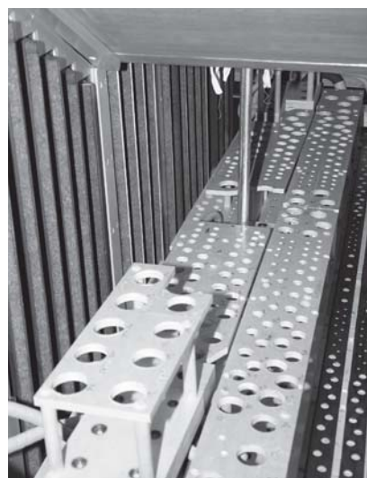
The interior of the Rückpositiv is ready for pipe installation (photo credit: Ron Turner)
